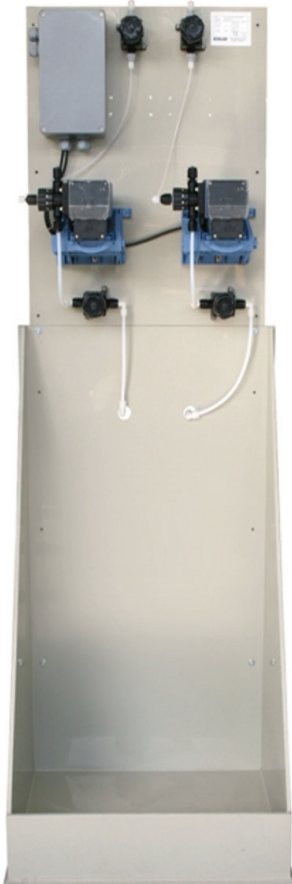
2 EMP KKS pumps 2 metering lines
