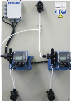
2 EMP KKS pumps, 1 metering line
